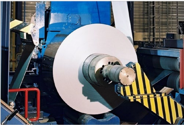
Condition monitoring of bearings
