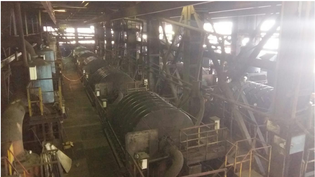
Slurry filtering through vacuum disc filters in Ukraine. A need of moisture measurement after each filters section.
