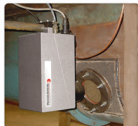
Moisture through sight glass
