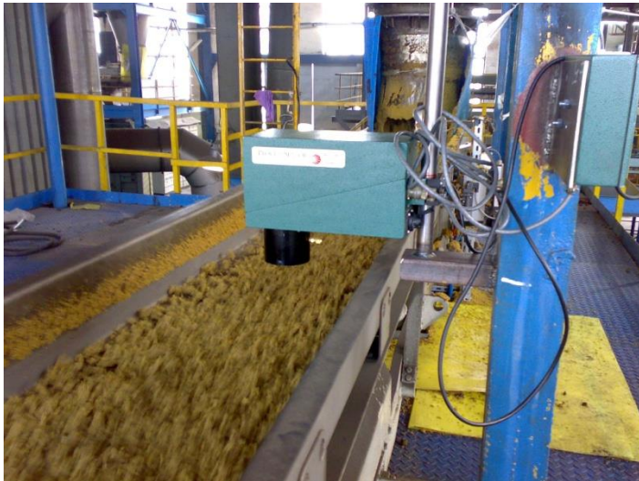
Moisture on open conveyors
