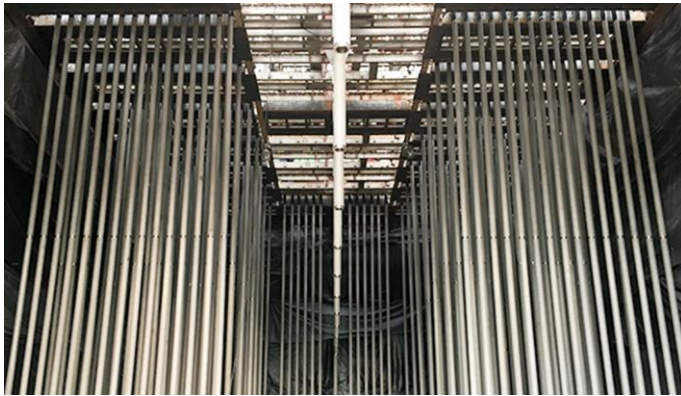
Steam reformer tubes
