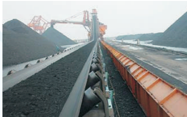
Mine Belt conveyors, air compressors, crushers, ball mills, centrifugal dehydrators and so on
